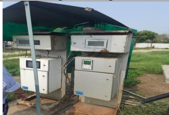
OCEMS installed at CETP Inlet (Defunct)
