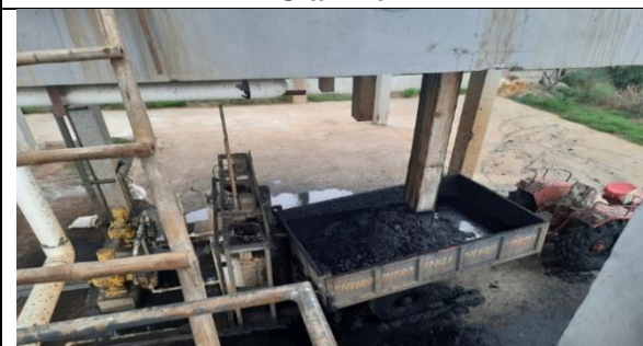
Collection of sludge in trolley
