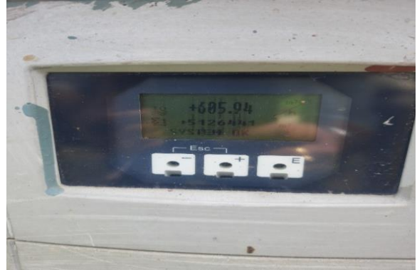
Flow meter installed at CETP Inlet
