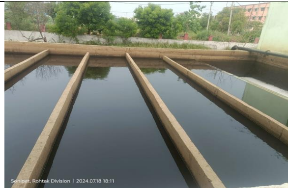
Chlorine Contact Tank
