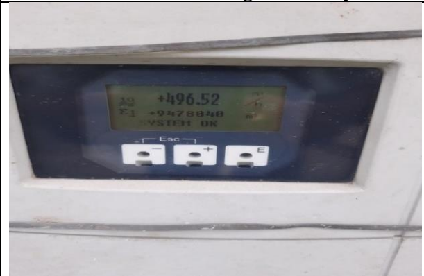
Flow meter installed at CETP Outlet
