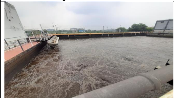
Aeration in SBR Tank
