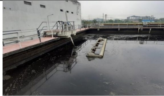
Decantation in SBR Tank
