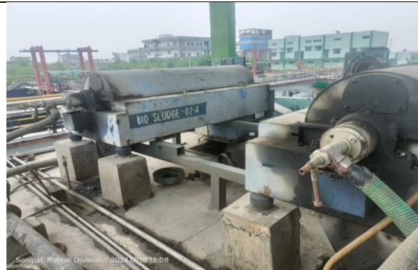
Sludge dewatering unit
