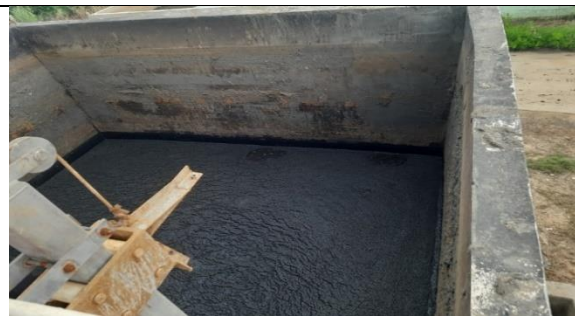
Sludge Holding Tank
